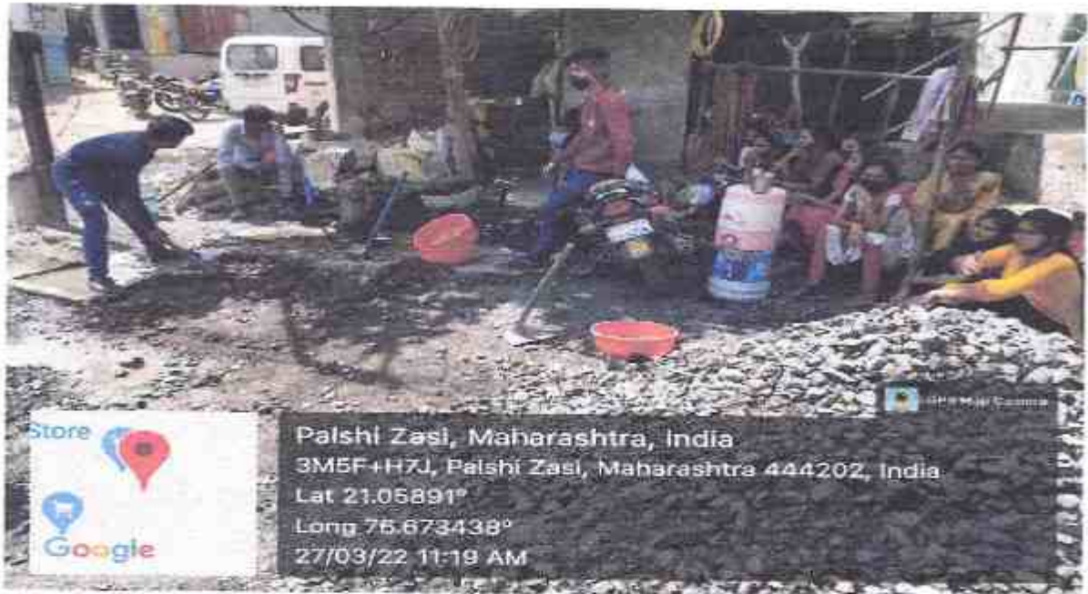
Absorption Pit at public tap is being dug by college students at village Palshi Jhashi on 27 th March, 2022
